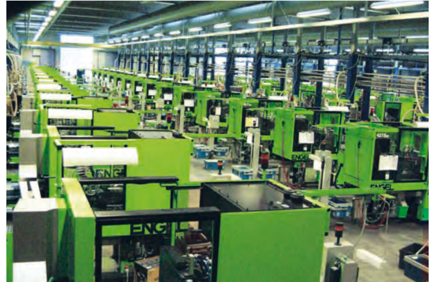
Partial view of a production plant with 64 ENGEL victory 330 / 75 type units for small precision parts
